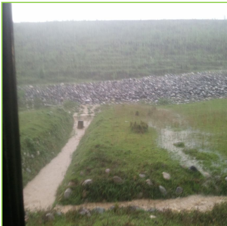
VIEW OF SEEPAGE DRAIN (MUDDY WATER COMES OUT)
